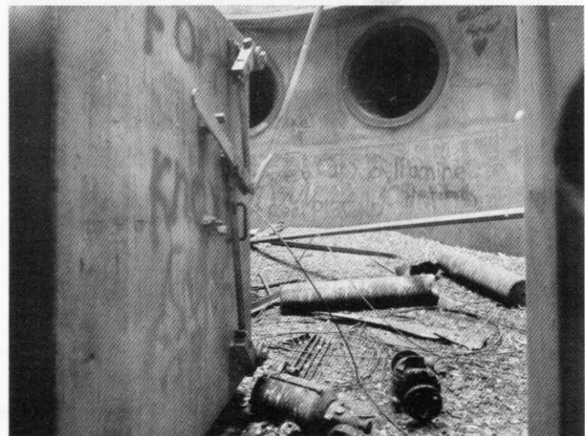
Looking through the personnel blast door into the exhaust shaft. The holes in the wall would originally have been covered by large blast valve closures
